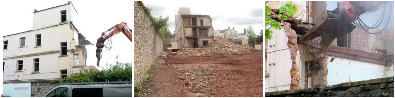
Above (L-R): L - Jurassic Park comes to Clifton! M – Progress on site, R – The machinery in action ‘eating’ it’s way through
