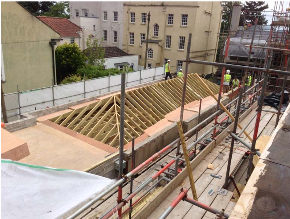
The above photograph shows the progress on the former stable block roof, with the roof now ready for felt, batten and slate tiles.
