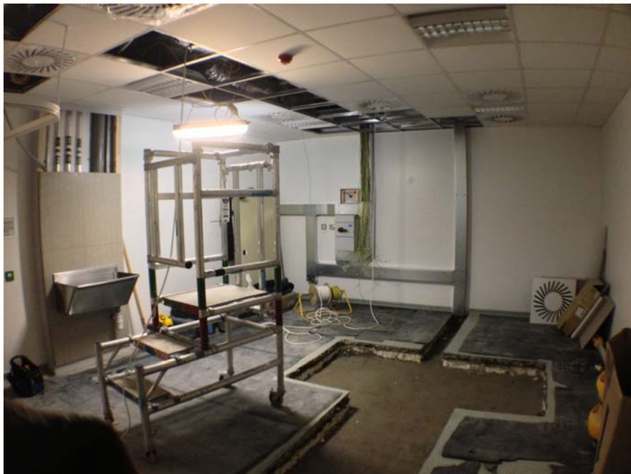
The above photograph shows the CT scanner room within the basement of the hospital building. The scanner will be located within the cut-out area in the floor.
